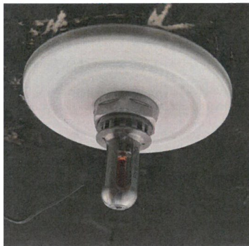
Figure 4 – Installed pendent nozzle
